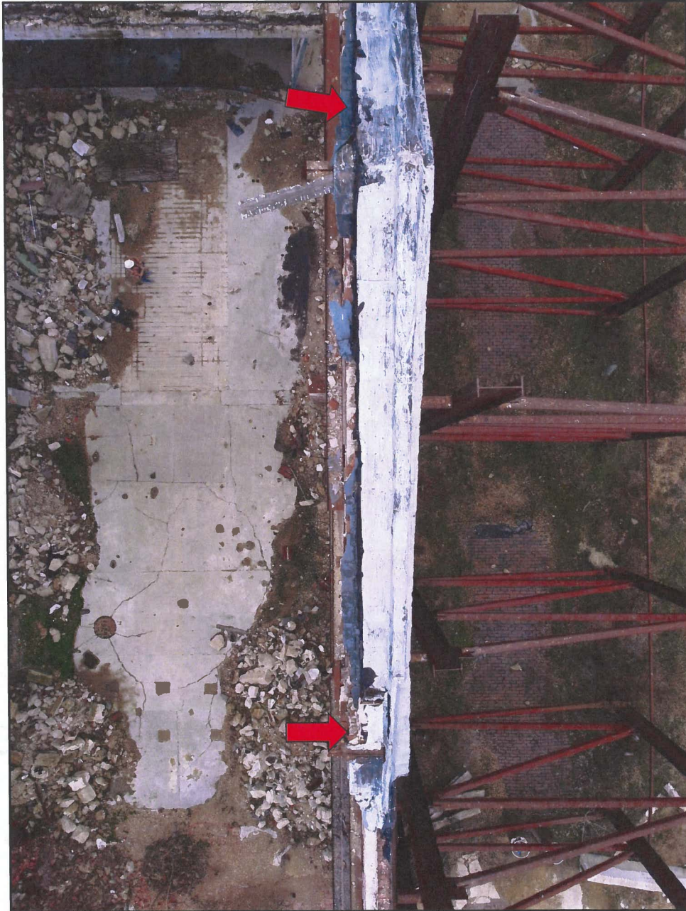
Photo 16 Hendler Building North Façade – Top Surface Above Pediment Note Missing Coping and Openings in Brick
