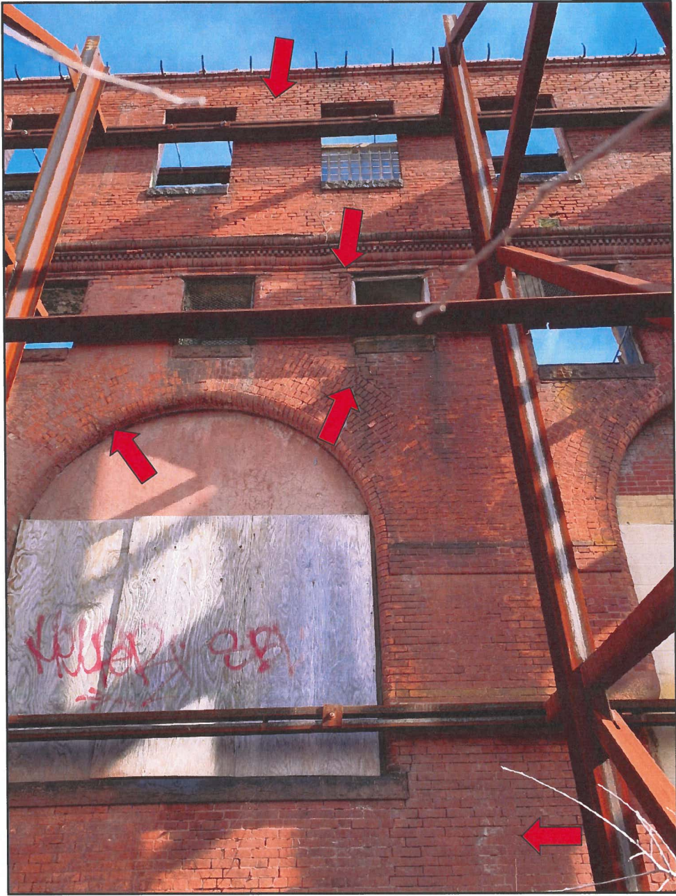
Photo 1 Hendler Building West Façade - Exterior Face Note Deteriorated Brick and Mortar Joints, Cracks, Bulge And Efflorescence
