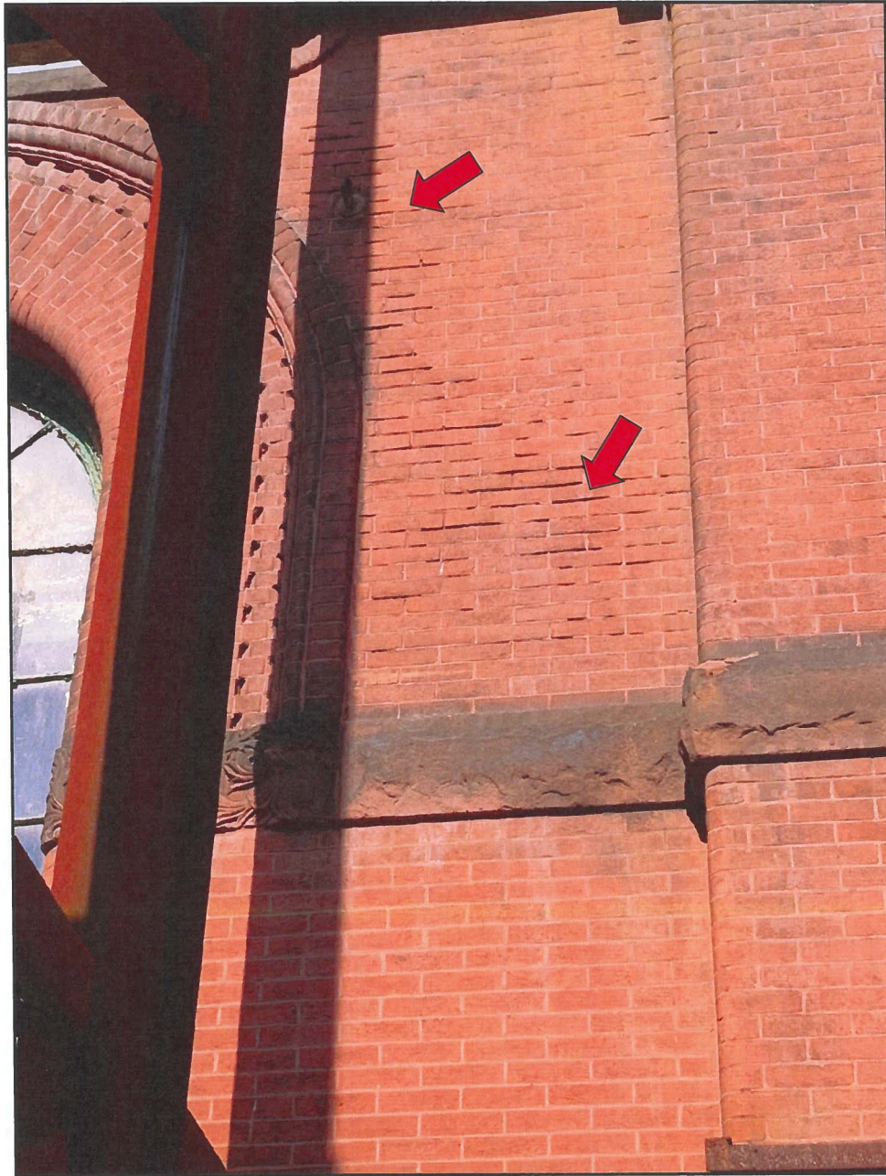
Photo 4 Hendler Building South Façade - Exterior Face Note Deteriorated Brick and Eroded Mortar Joints
