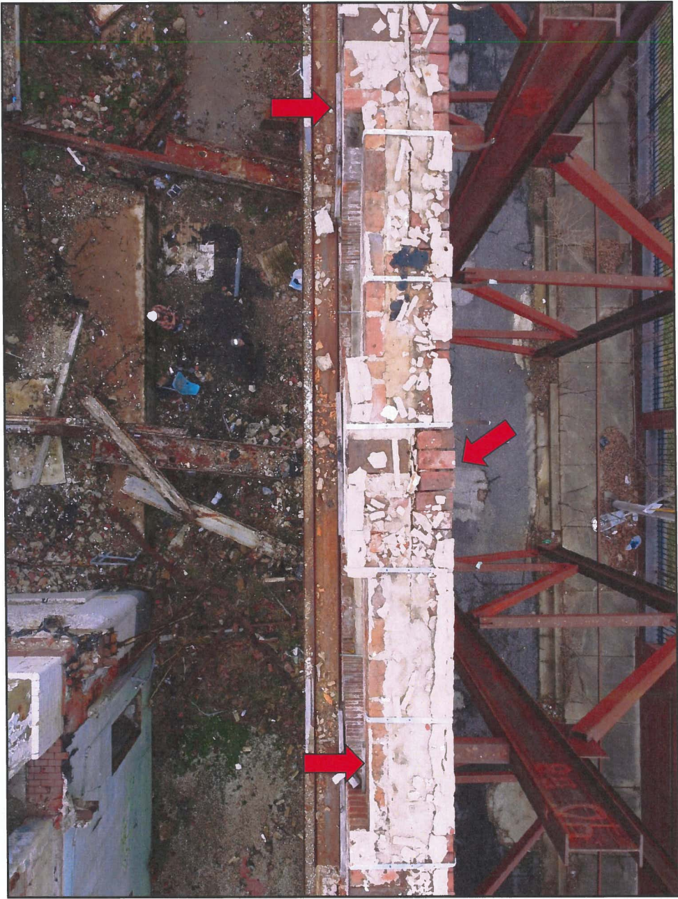
Photo 18 Hendler Building West Façade – Top Surface Note Missing Coping and Openings in Brick
