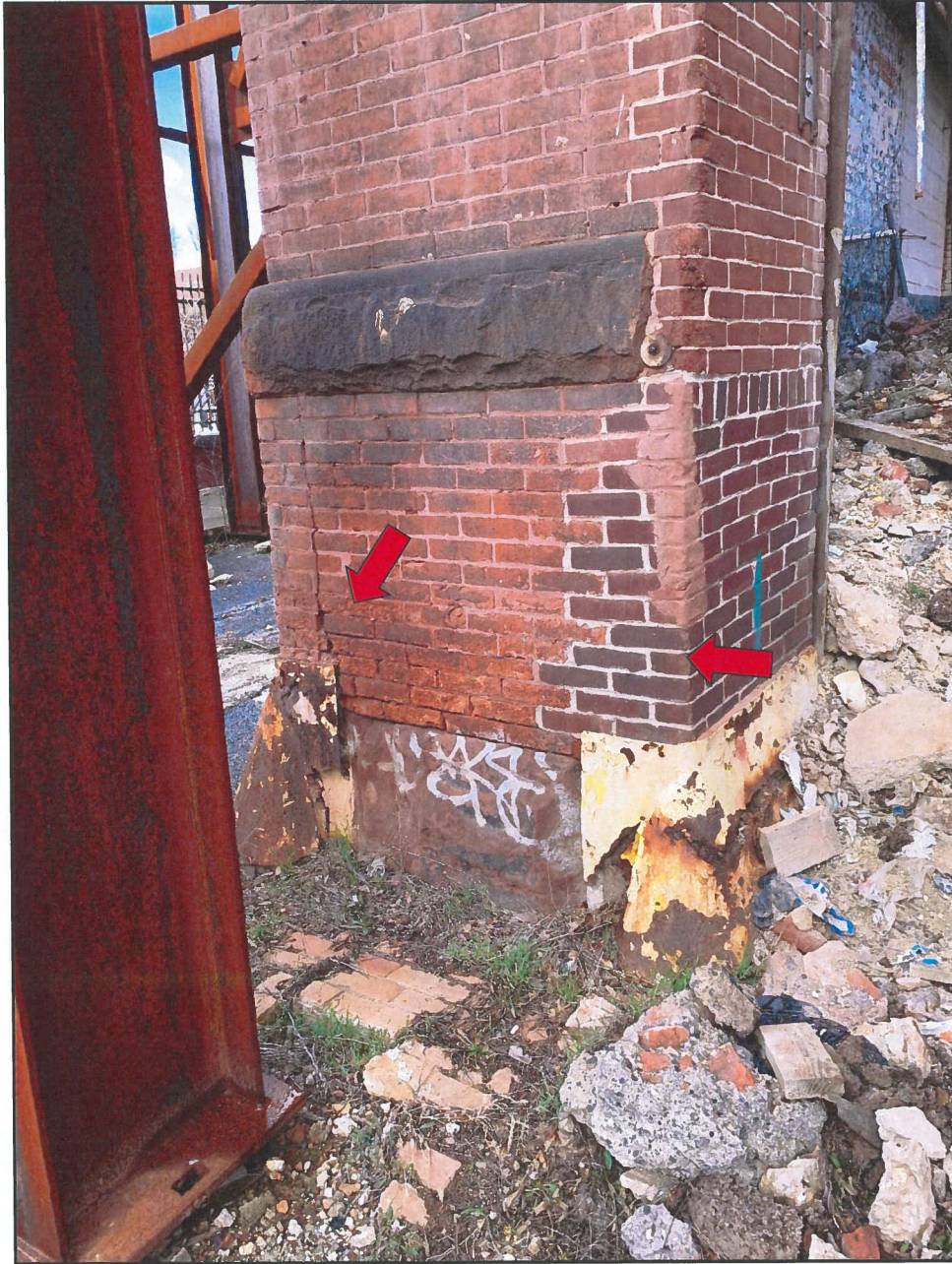
Photo 6 Hendler Building South Façade - Exterior Face Note Deteriorated Brick and Eroded Mortar Joints Cracks and Prior Repairs
