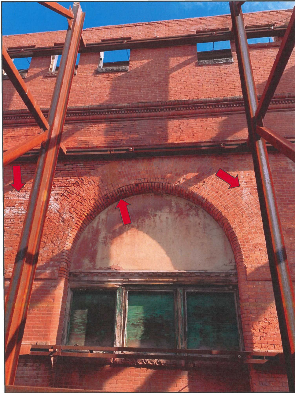
Photo 5 Hendler Building West Façade - Exterior Face Note Severely Deteriorated Brick and Mortar Joints, and Efflorescence
