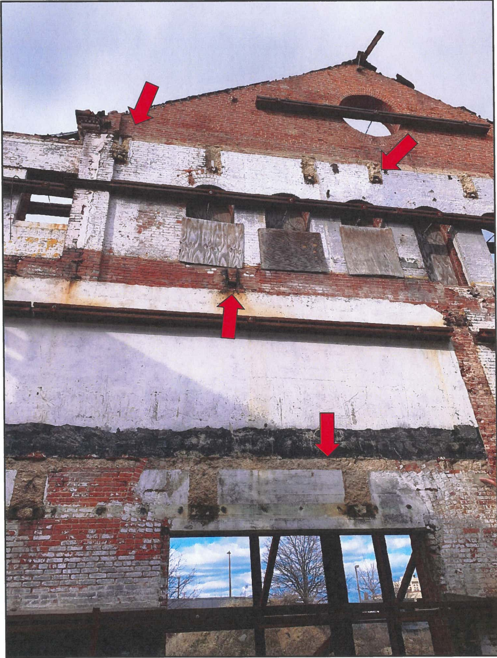
Photo 11 Hendler Building North Façade - Interior Face Note Openings in Brick, Beam Pockets and Embedded Concrete Floor
