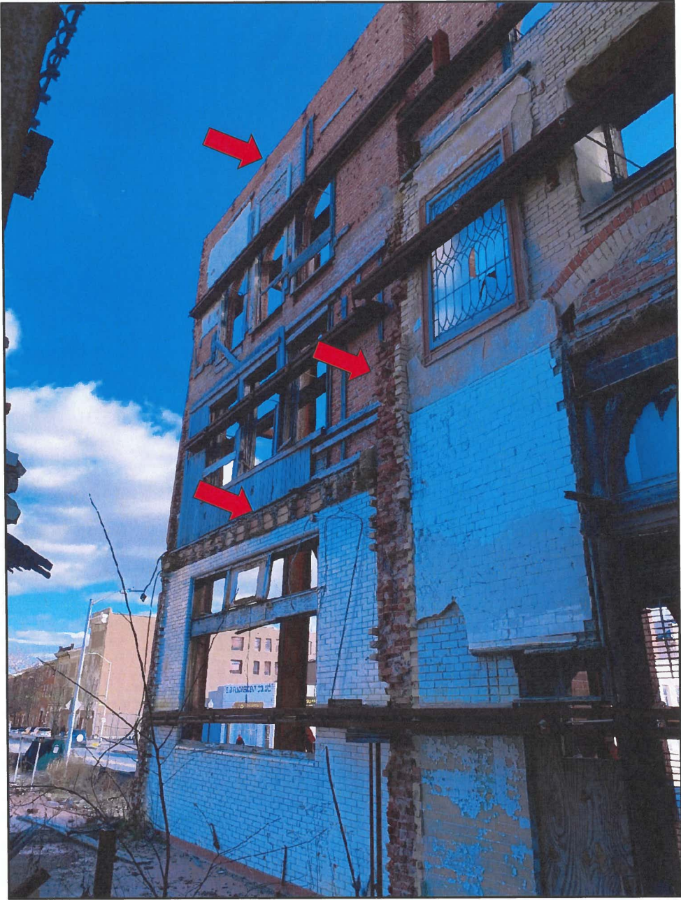
Photo 8 Hendler Building South Façade - Interior Face Note Openings in Brick, Beam Pockets and Embedded Concrete Floor
