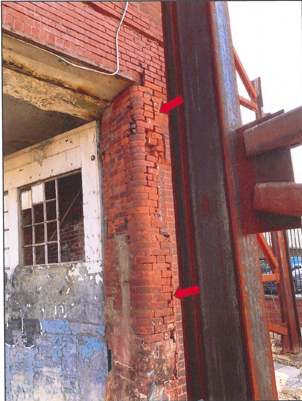
Photo 3 Hendler Building North Façade - Exterior Face Note Deteriorated Brick and Eroded Mortar Joints and Cracks
