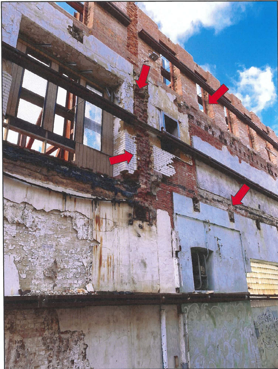
Photo 11 Hendler Building West Façade - Interior Face Note Openings in Brick, Beam Pockets and Missing Window Frames
