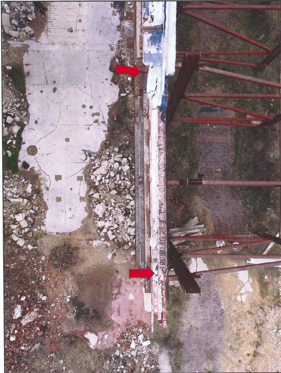
Photo 17 Hendler Building North Façade – Top Surface Note Missing Coping and Openings in Brick
