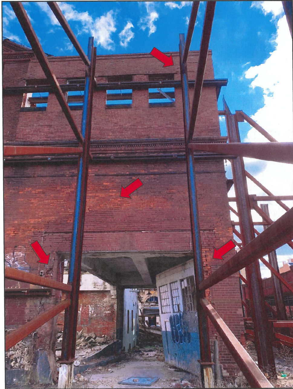
Photo 1 Hendler Building North Façade - Exterior Face Note Deteriorated Brick and Eroded Mortar Joints and Cracks
