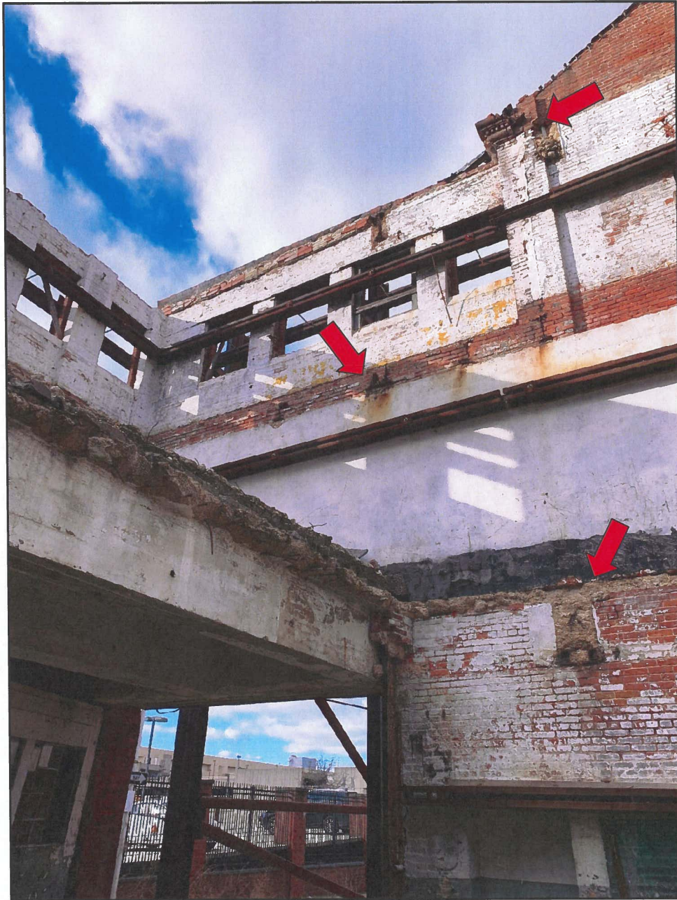
Photo 10 Hendler Building North Façade - Interior Face Note Openings in Brick, Beam Pockets and Embedded Concrete Floor
