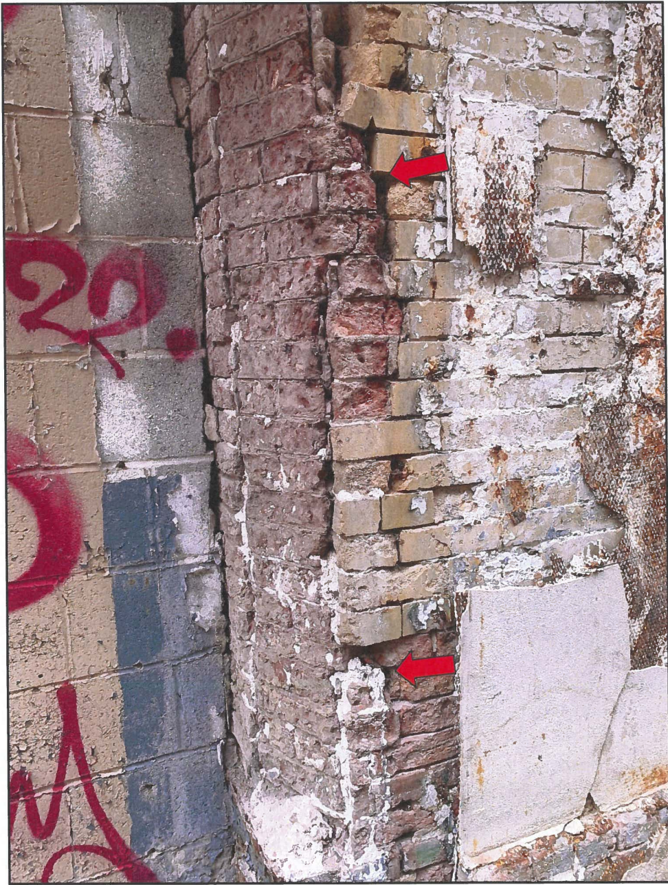
Photo 14 Hendler Building West Façade - Interior Face Note Severely Deteriorated Brick and Mortar Joints
