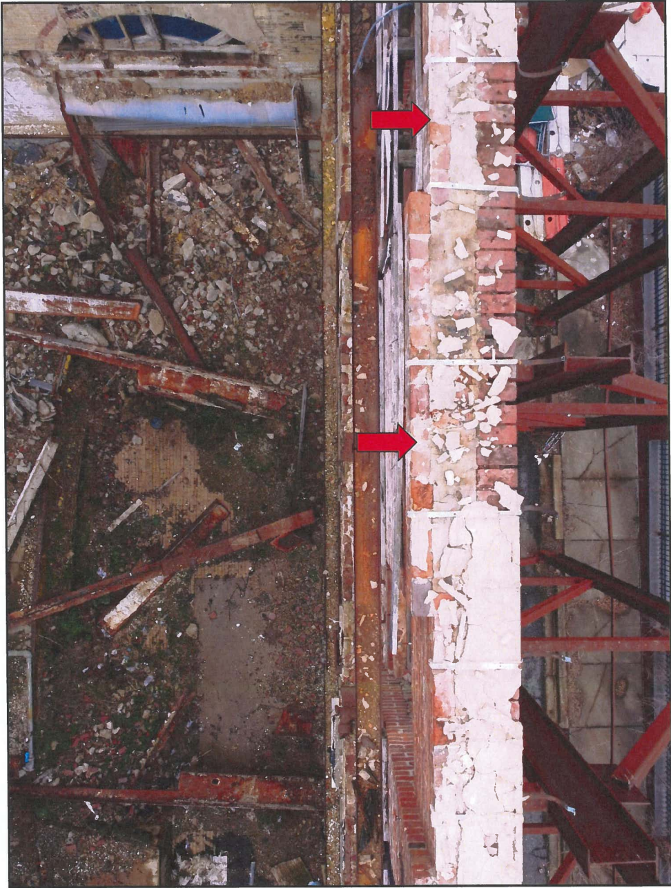
Photo 16 Hendler Building West Façade – Top Surface Note Missing Coping and Openings in Brick
