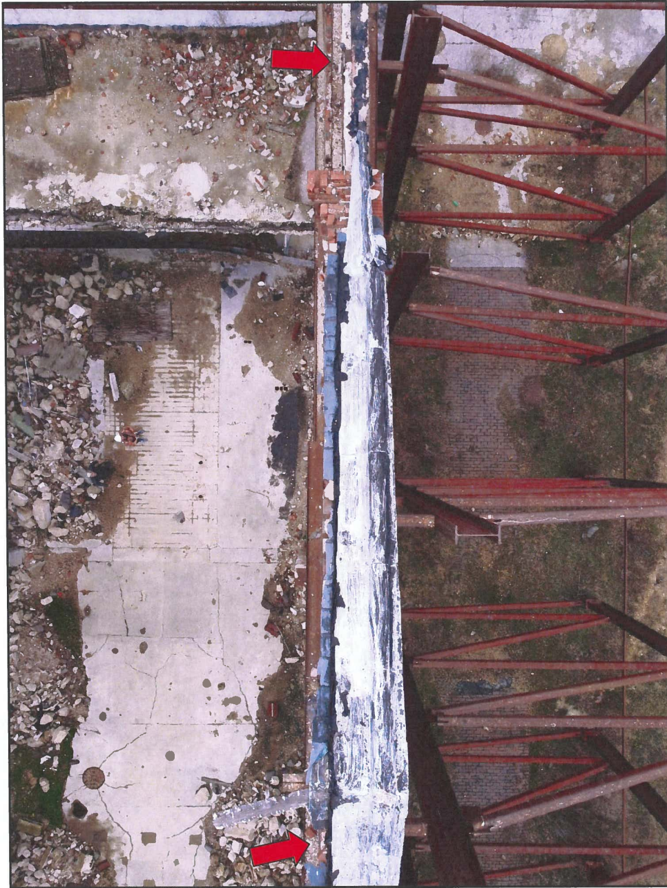
Photo 15 Hendler Building North Façade – Top Surface Above Pediment Note Missing Coping and Openings in Brick
