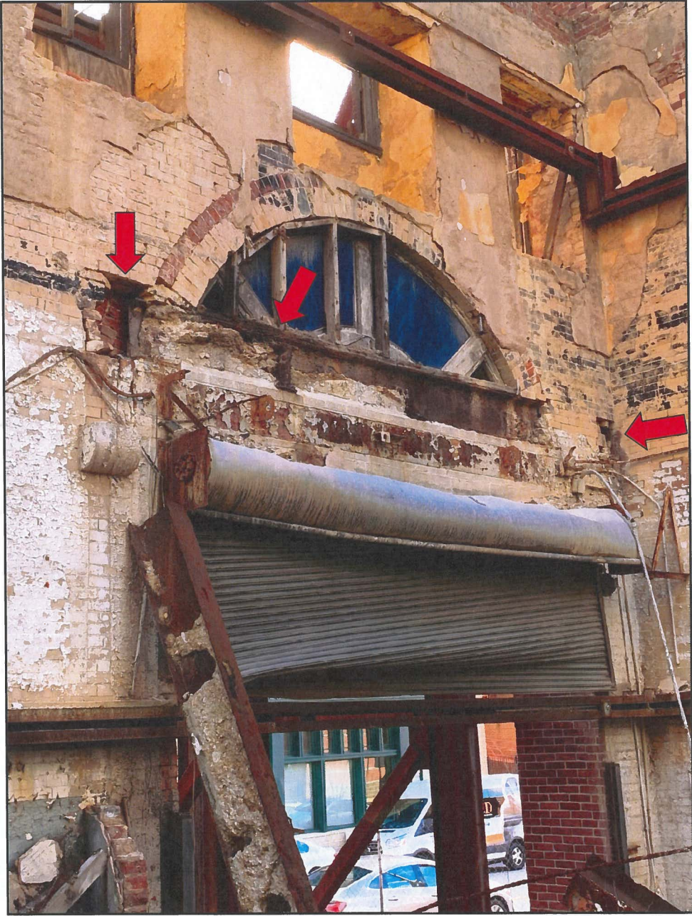
Photo 13 Hendler Building South Façade - Interior Face Note Openings in Brick and Embedded Beam with Pack Rust
