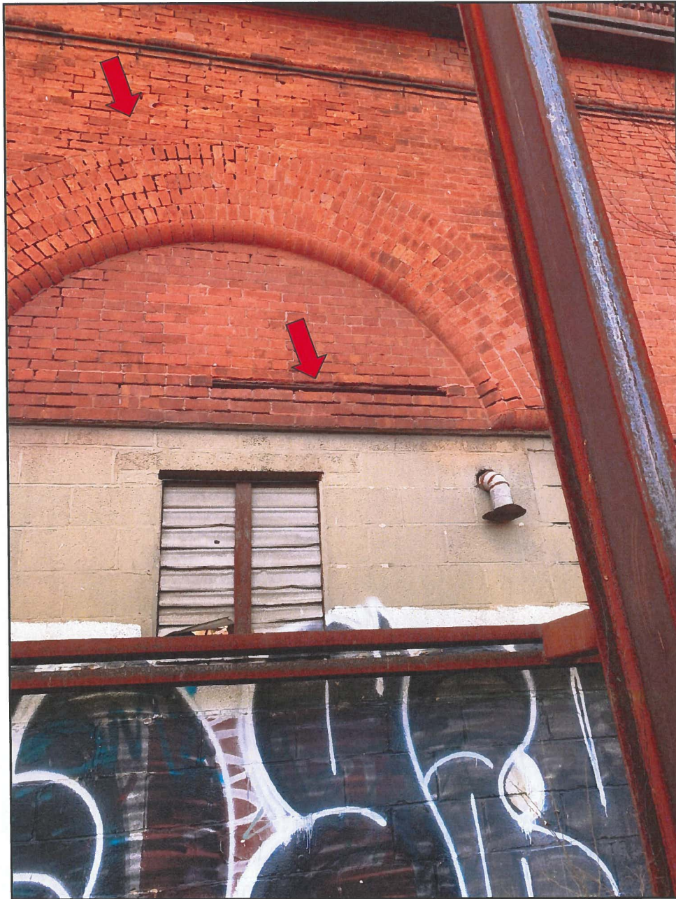
Photo 5 Hendler Building North Façade - Exterior Face Note Deteriorated Brick and Eroded Mortar Joints, and Deteriorated Lintel with Pack Rust
