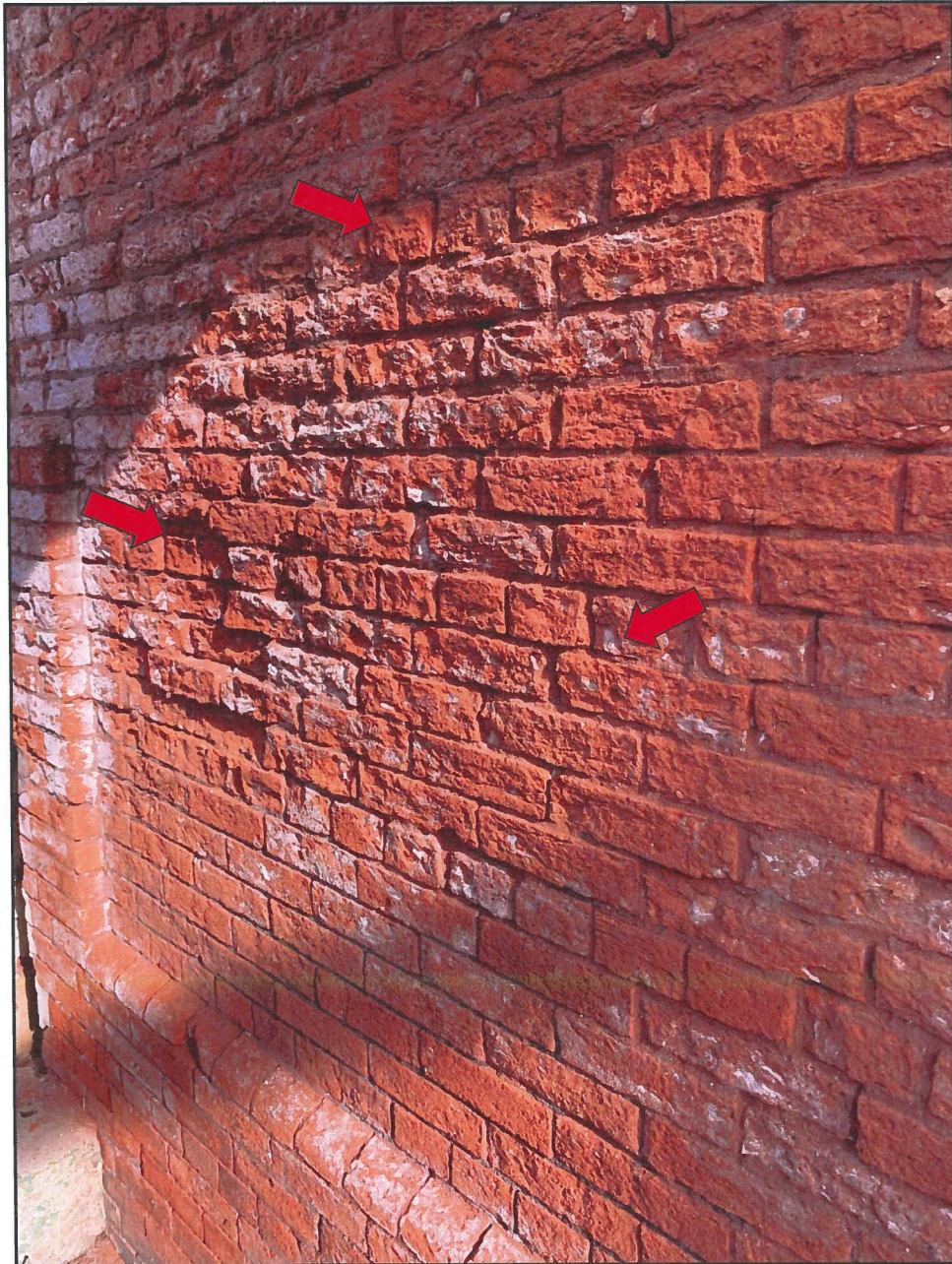
Photo 8 Hendler Building West Façade - Exterior Face Note Severely Deteriorated Brick and Mortar Joints, and Efflorescence
