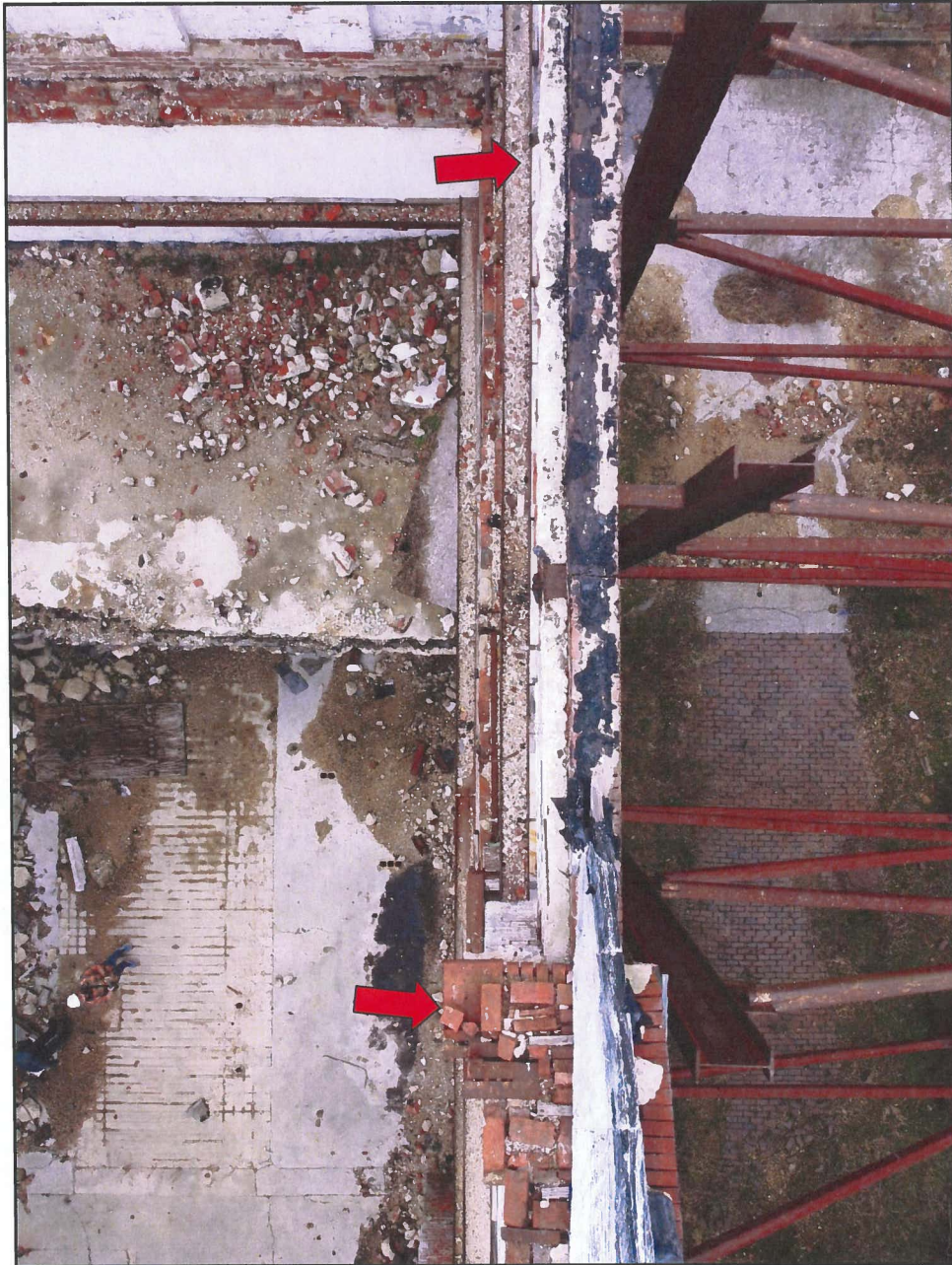
Photo 14 Hendler Building North Façade – Top Surface Note Missing Coping and Openings in Brick
