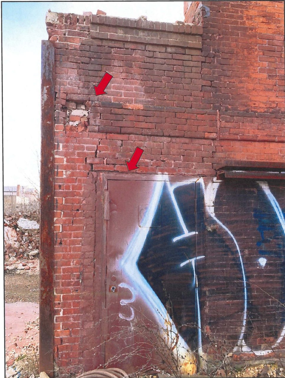
Photo 6 Hendler Building North Façade - Exterior Face Note Deteriorated Brick and Eroded Mortar Joints, and Deteriorated Lintel with Pack Rust
