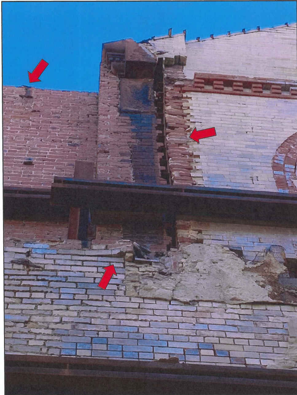
Photo 9 Hendler Building South Façade - Interior Face Note Openings in Brick, Beam Pockets, Eroded Mortar and Loose Brick
