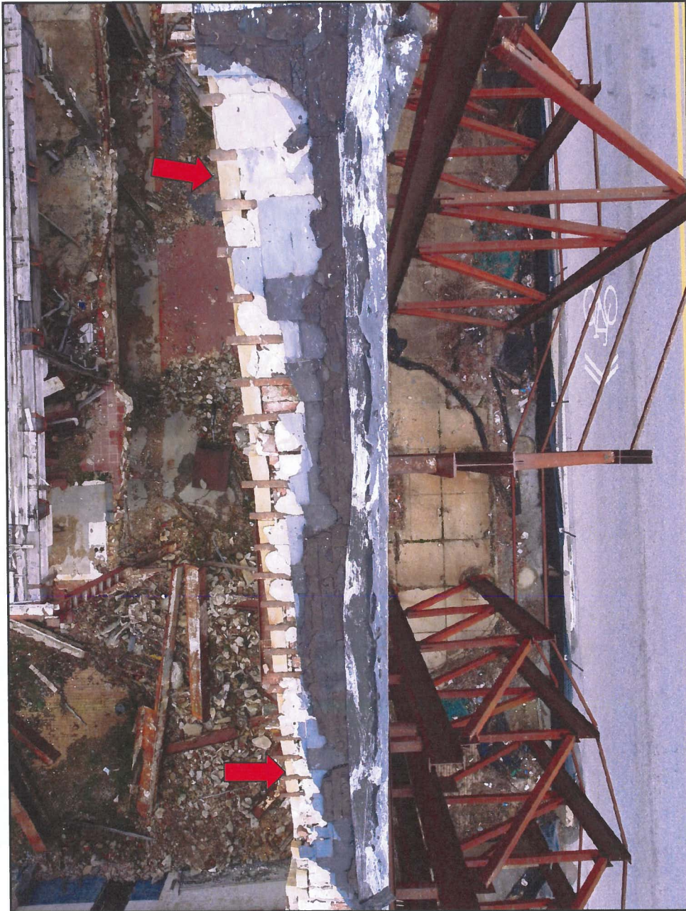
Photo 17 Hendler Building South Façade – Top Surface Above Pediment Note Missing Coping and Openings in Brick
