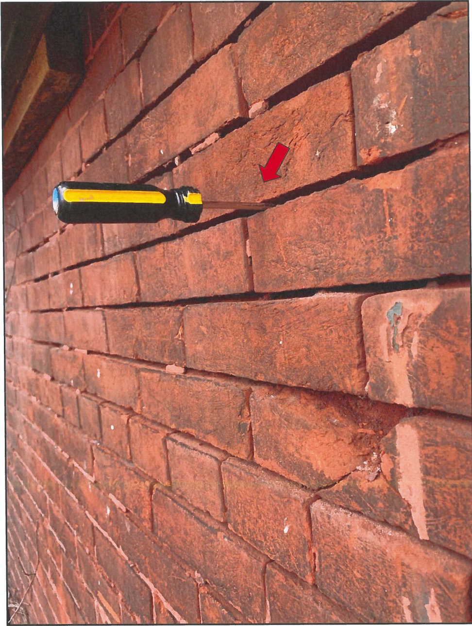
Photo 7 Hendler Building North Façade - Exterior Face Note Deteriorated Brick and Eroded Mortar Joints, Screwdriver Inserted to 3" Depth
