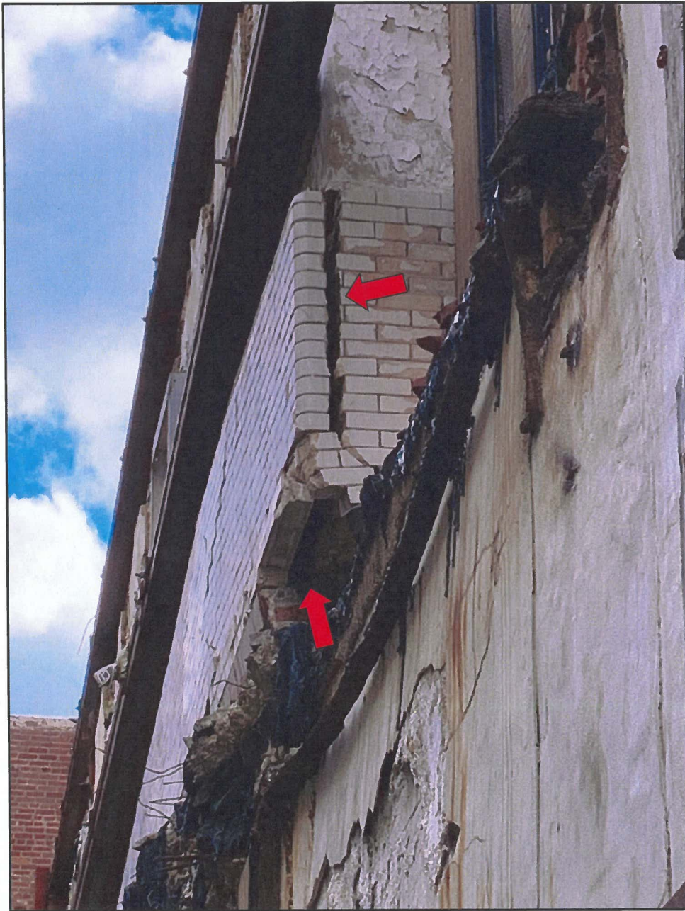
Photo 12 Hendler Building West Façade - Interior Face Note Large Crack and Unsupported Brick Veneer
