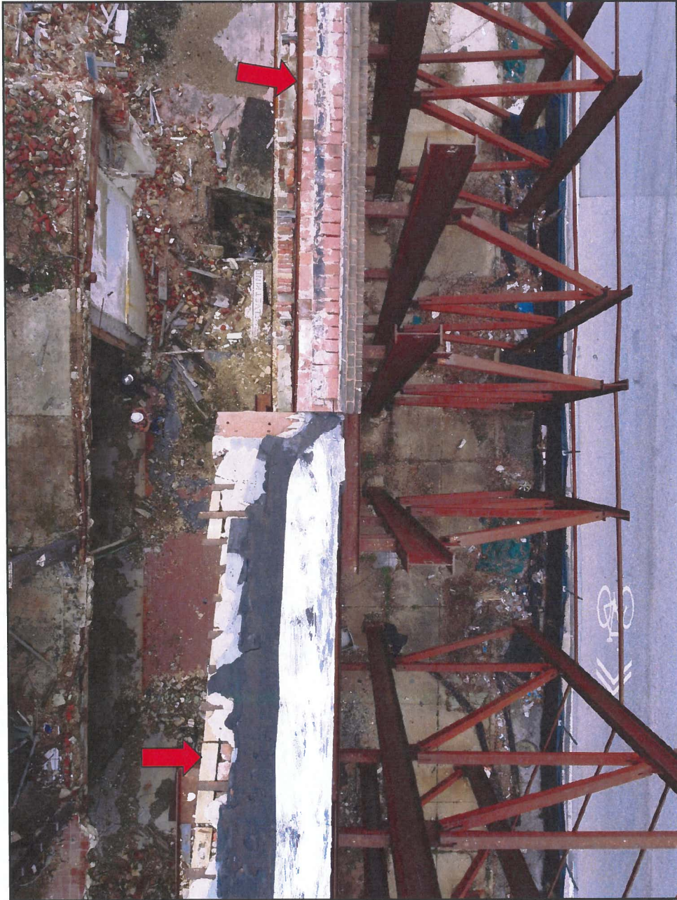
Photo 16 Hendler Building South Façade – Top Surface Above Pediment Note Missing Coping and Openings in Brick
