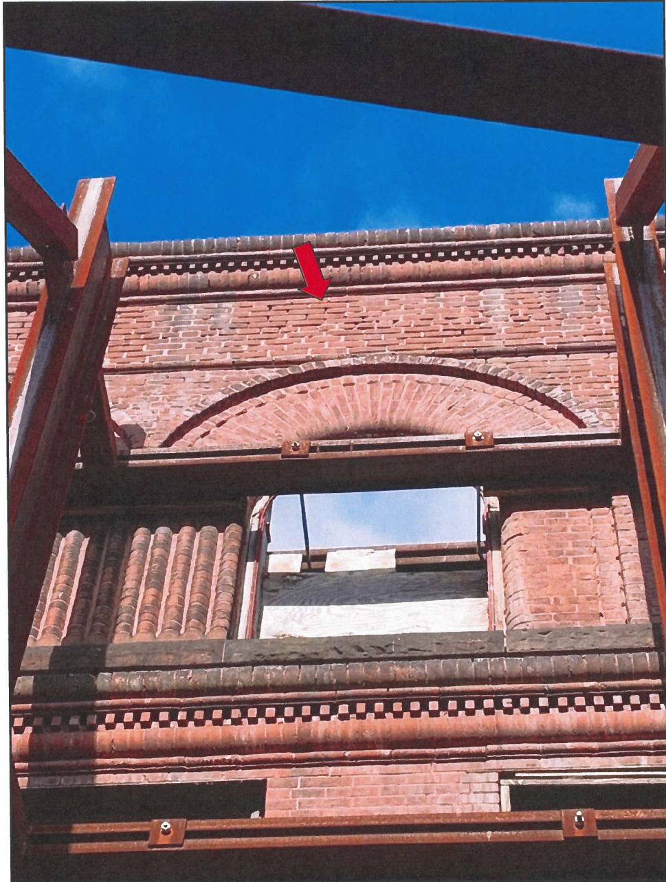
Photo 5 Hendler Building South Façade - Exterior Face Note Deteriorated Brick and Eroded Mortar Joints
