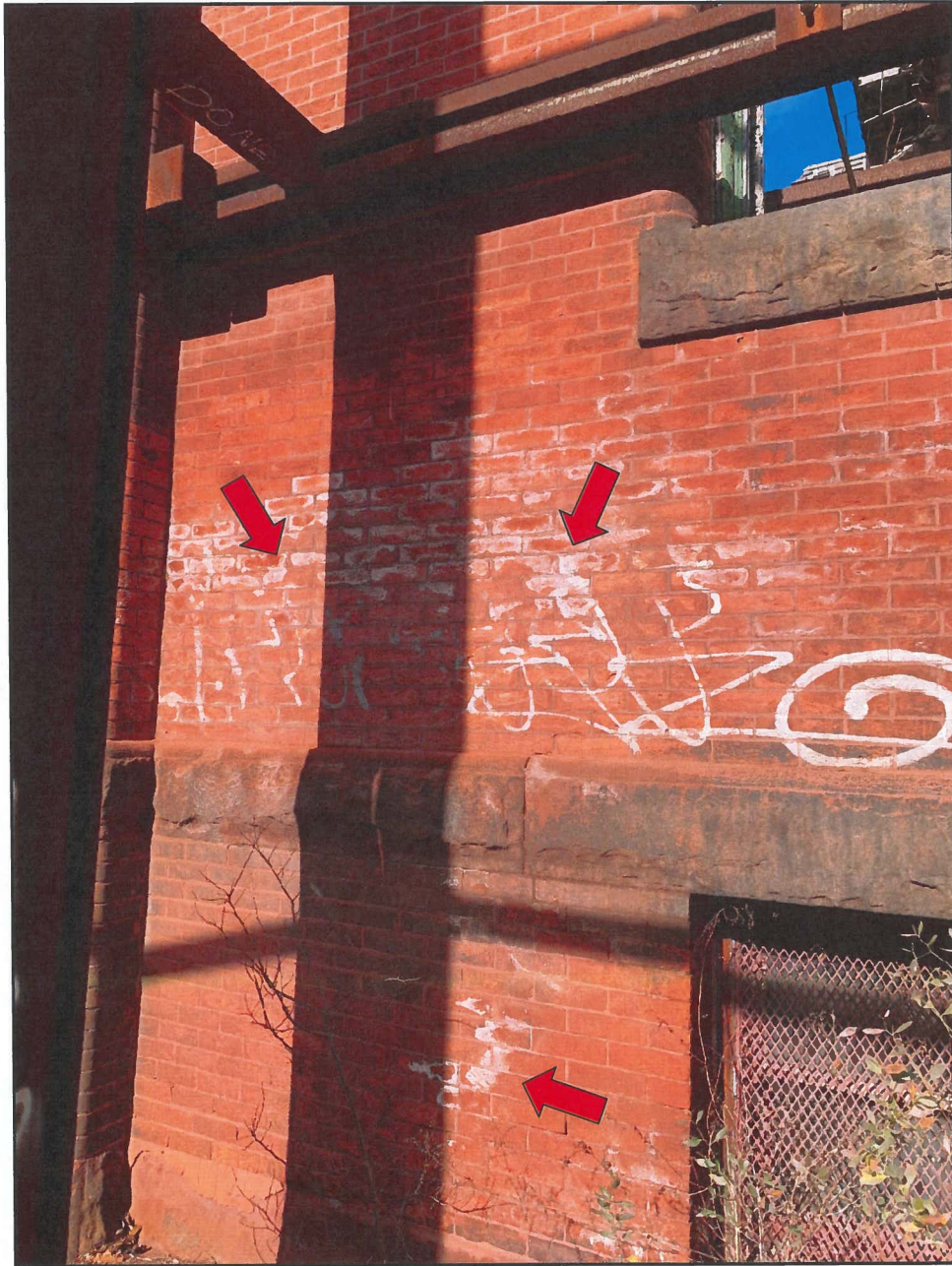
Photo 1 Hendler Building South Façade - Exterior Face Note Efflorescence on Wall
