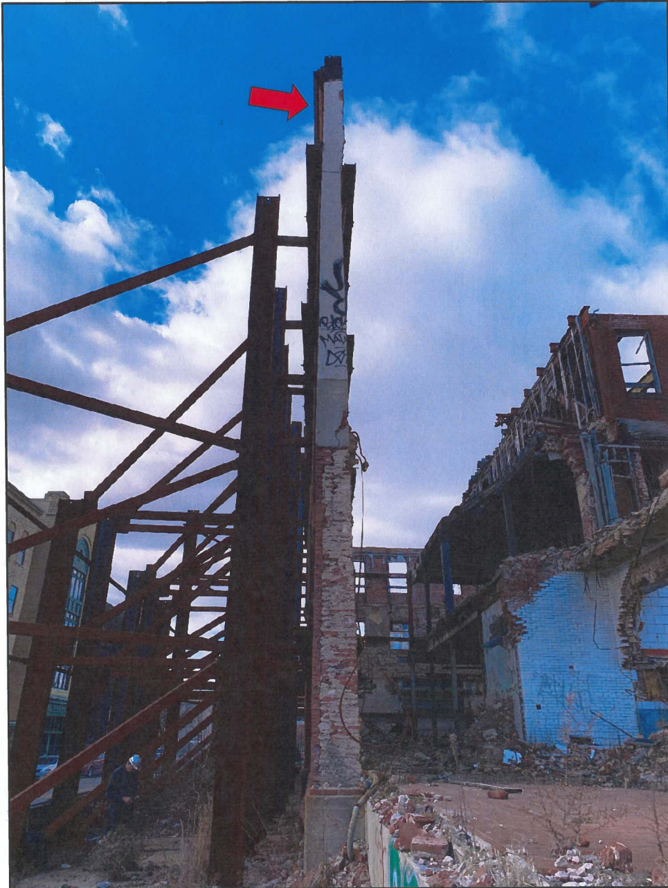
Photo 7 Hendler Building South Façade - Exterior Face Note Lean in Upper Section of Façade
