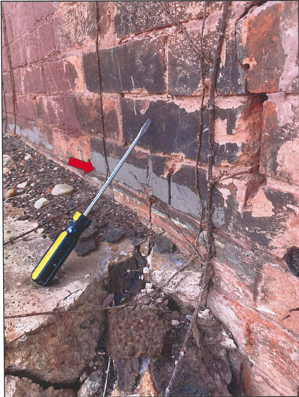
Photo 9 Hendler Building North Façade - Exterior Face Note ¼" Diameter x 6" Long Screwdriver That Was Used to Probe Mortar Joints
