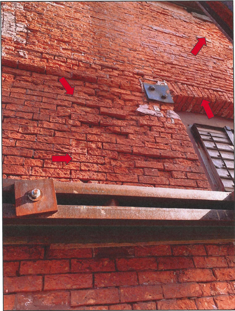
Photo 10 Hendler Building West Façade - Exterior Face Note Severely Deteriorated Brick and Mortar Joints
