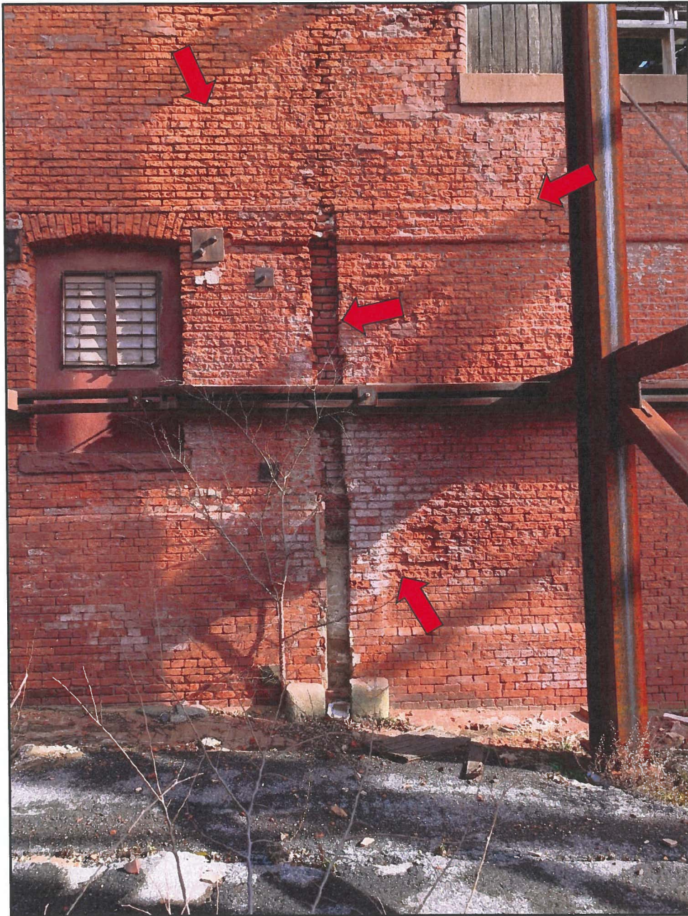
Photo 9 Hendler Building West Façade - Exterior Face Note Severely Deteriorated Brick and Mortar Joints, Cracks Slot in Wall and Efflorescence
