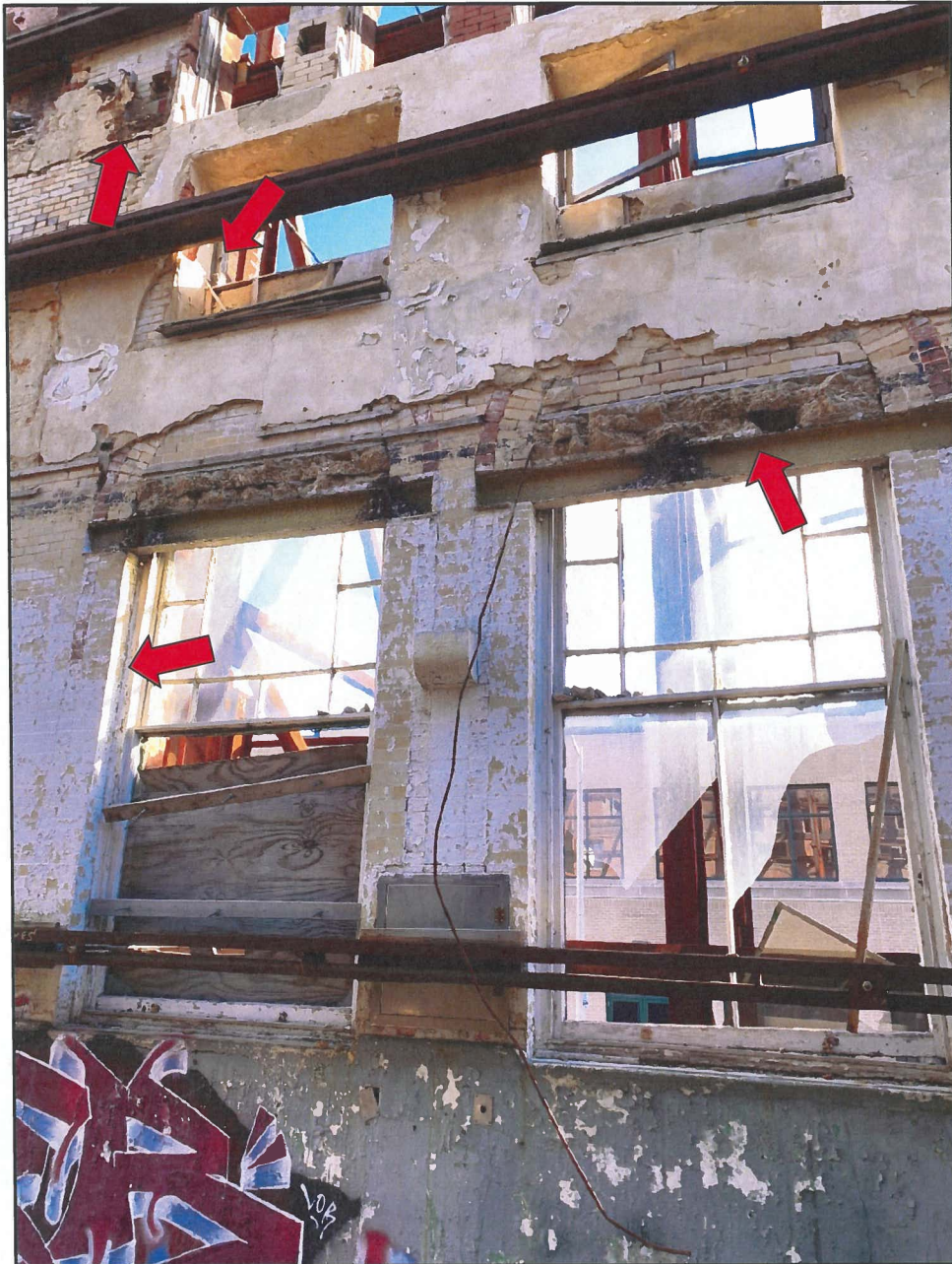
Photo 10 Hendler Building South Façade - Interior Face Note Openings in Brick, Missing or Deteriorated Window Frames and Embedded Concrete Floor
