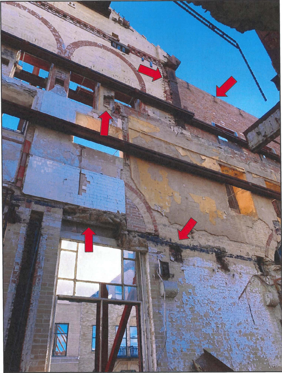
Photo 11 Hendler Building South Façade - Interior Face Note Openings in Brick, Beam Pockets and Embedded Concrete Floor
