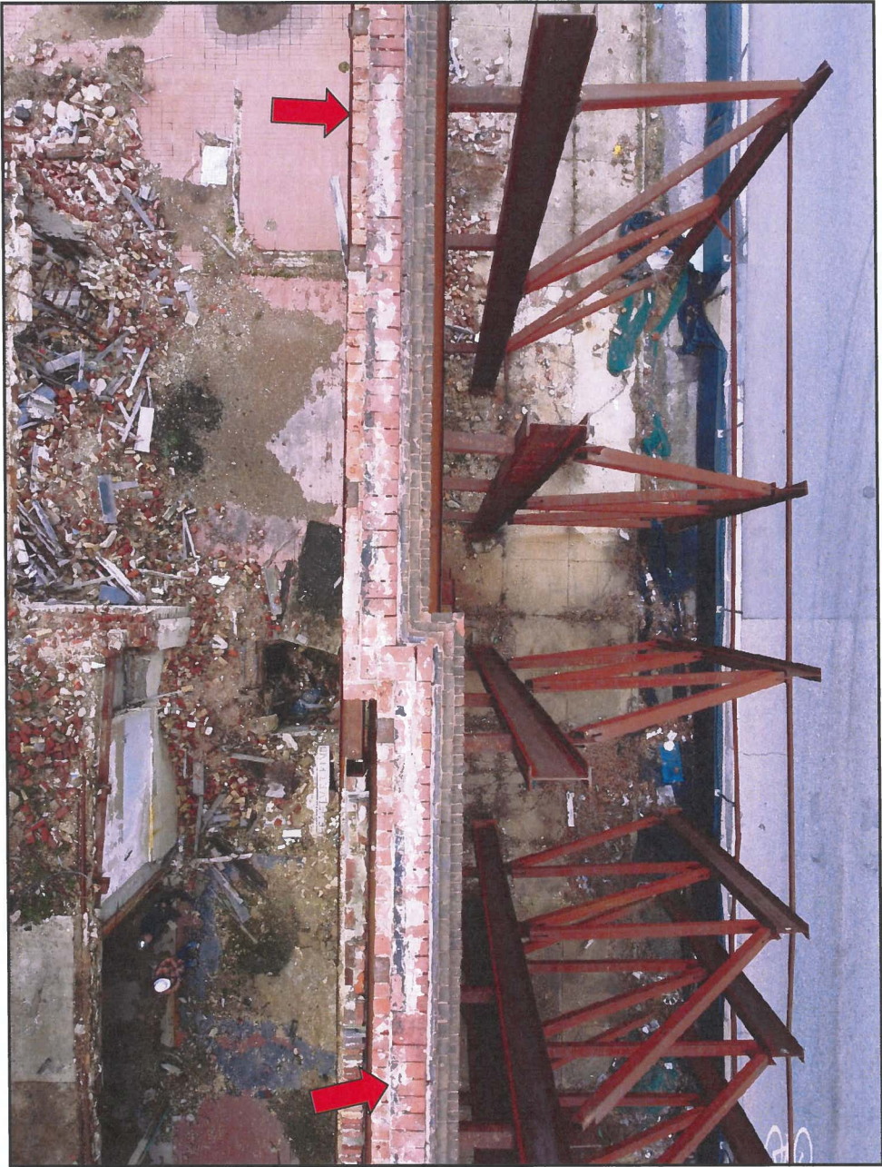
Photo 15 Hendler Building South Façade – Top Surface Note Missing Coping and Openings in Brick
