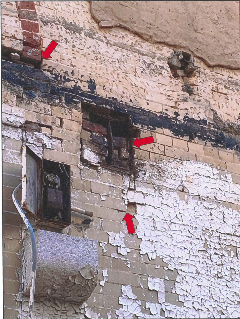
Photo 12 Hendler Building South Façade - Interior Face Note Openings in Brick, Embedded Beam with Pack Rust and Spalled Brick
